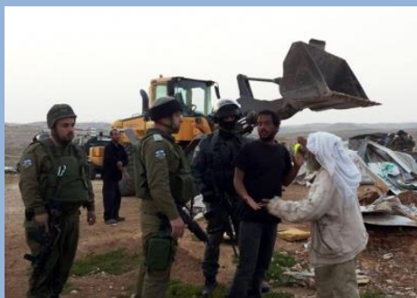
Residents of Um al-Kheir in the South Hebron Hills, against the backdrop of a bulldozer destroying structures in the community. Photo: Nasser Nawaj'ah, B'Tselem, 6 April 2016.
