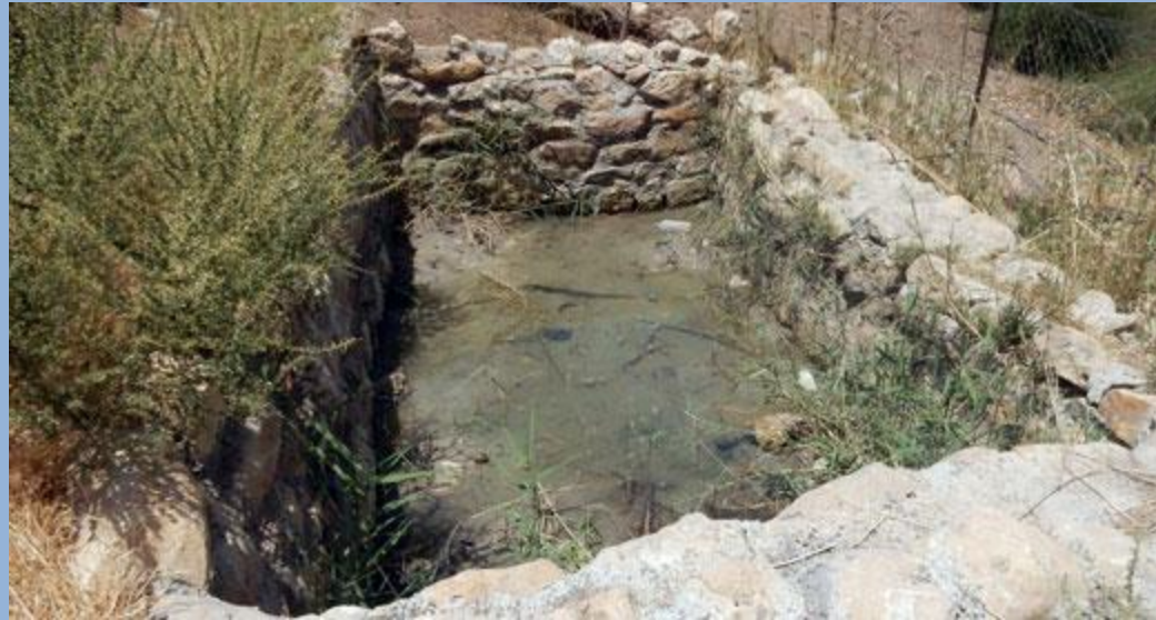
Spring water reservoir slated for demolition in Khirbet al-Malih. Photo: 'Aref Daraghmeh, B'Tselem, 14 June 2016
